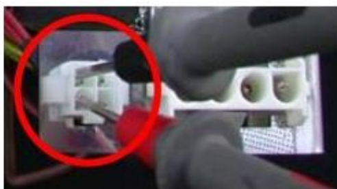
NTC sensor Boiler 2
